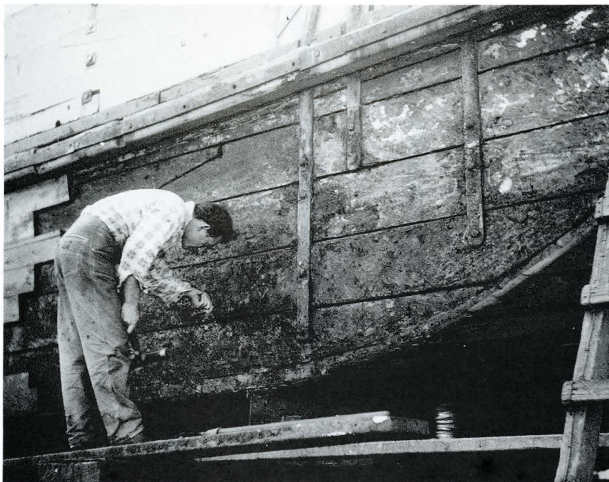
Caulking seams at the fore chainplates of the KOHI built as the CAED-MILE-FAILTE (G. Niccol, Auckland, 1911; 92.6 x 27.6 4.2 ft). The totara worm-sheathing has been stripped back. Note the junction of bow and side planking at the shoulder. (C.W. Hawkins)
